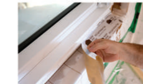
Fig 8.0 The installer has folded back the 12mm strip before removing the release liner
