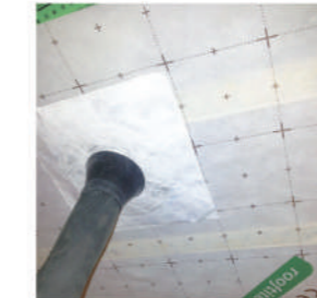
Fig 9.0 A solar pipe penetrating the membrane.
