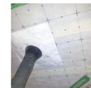
Fig 9.0 A solar pipe penetrating the membrane.
